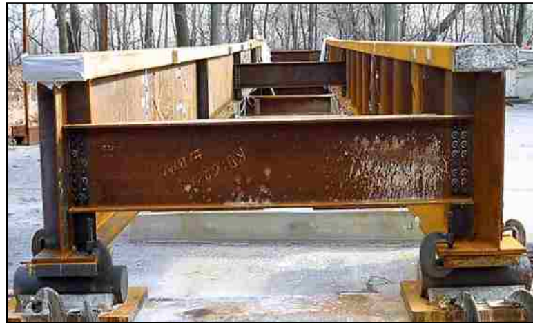
Figure 2.2: Straight TFGs with concrete-filled rectangular steel tube top flange (Wimer and Sause, 2004)
